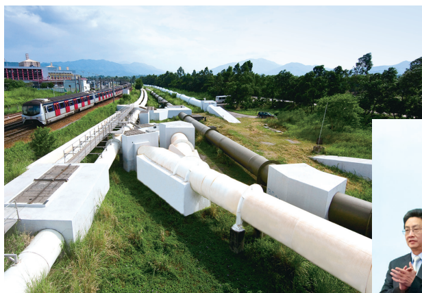
東江輸水管道 Raw Water Supply Pipeworks from Dongjiang
