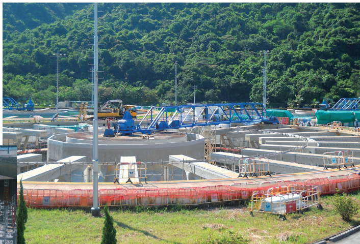
沙田濾水廠之澄清池 Clarifier at Sha Tin Water Treatment Works
