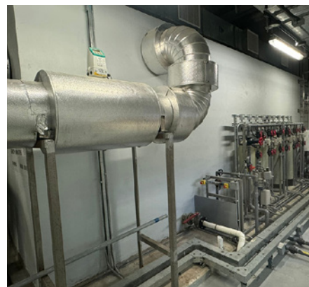
為雨水回收池而設的水管 Pipe arrangement for rainwater collection tank
