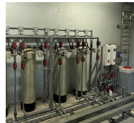
薄膜池 Membrane tank
